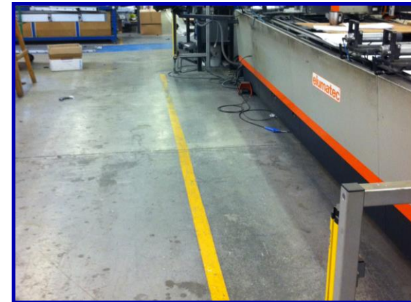
Sufficient safety devices are in place for high risk machines
