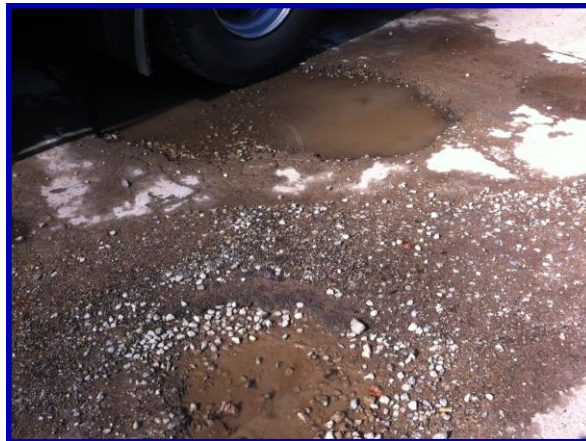
Pot holes in the delivery area must be repaired
